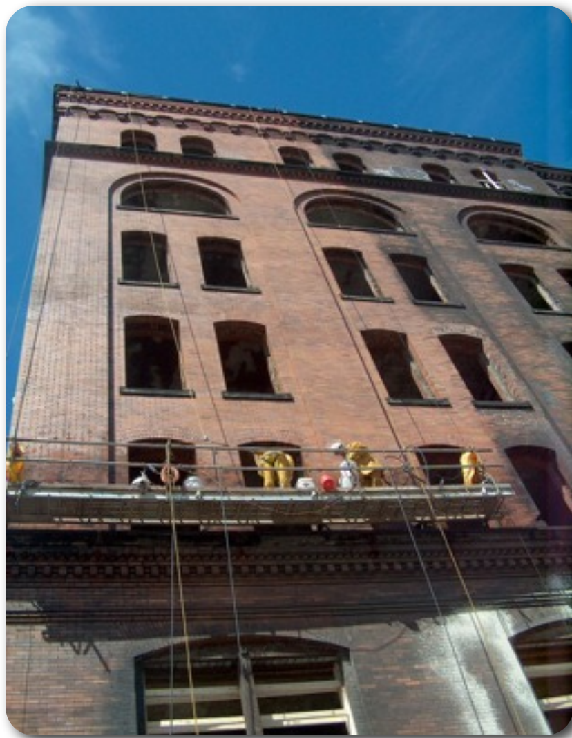
Restoration of the Armstrong Cork Factory was made possible in part by the federal Historic Preservation Tax Credit.
